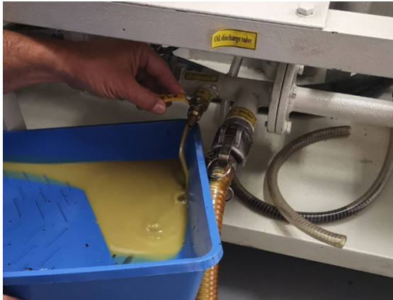
Figure 28. Drainage of the hydraulic oil before sampling
